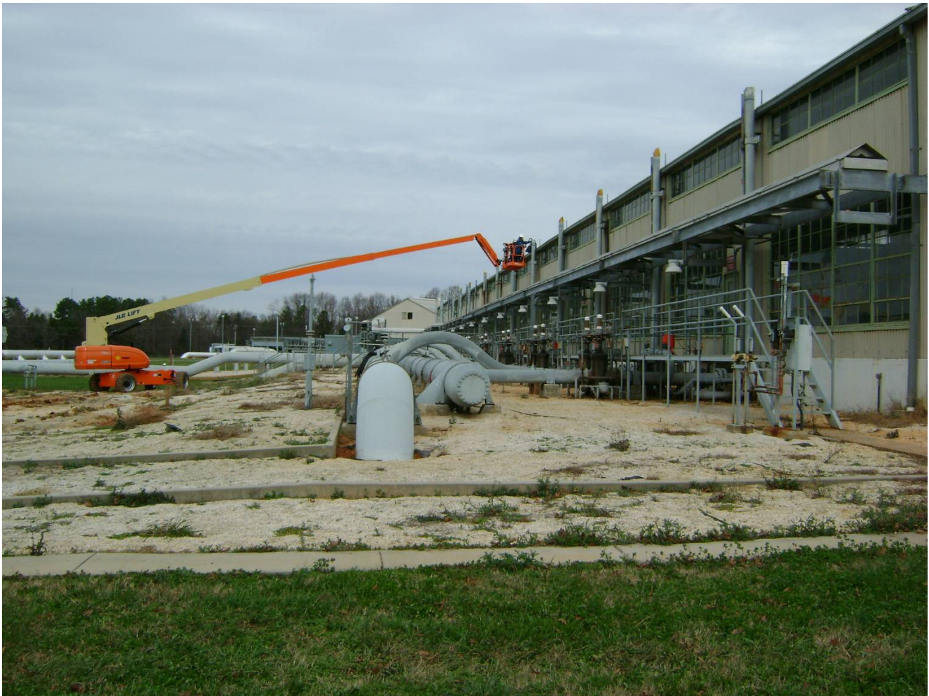
Figure 1. Manlift Use for Roofline Vent Access Can Introduce Significant Safety Concerns.
