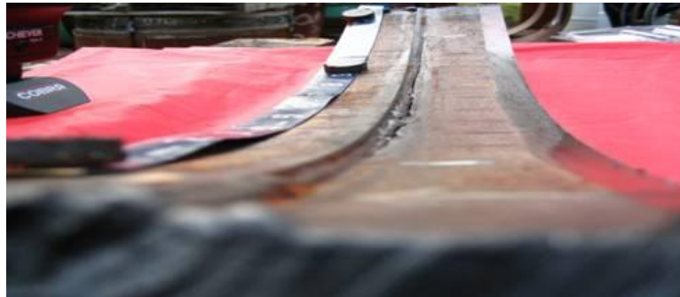
Figure 83. High-low misalignment with inadequate backweld
