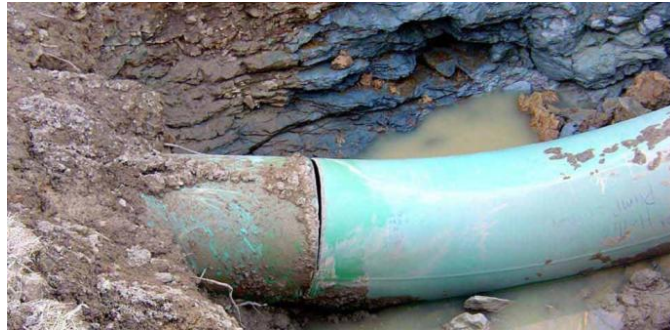
Figure B5. Girth weld failure at unequal-wall-thickness transition
