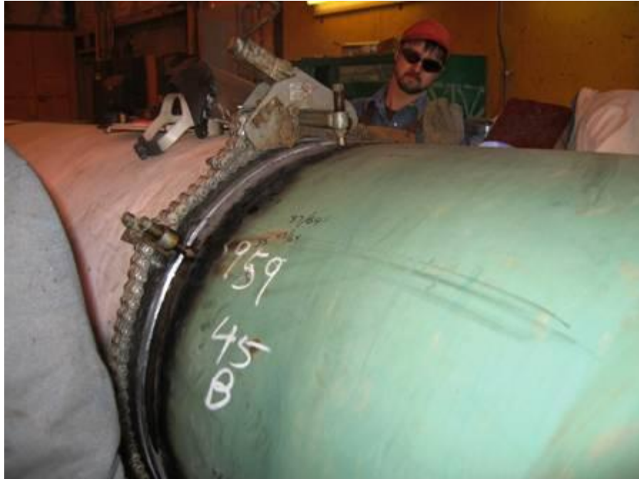
Figure 33. Temporary alignment of segmented bend to pipe pup section using Dearman-style clamp
